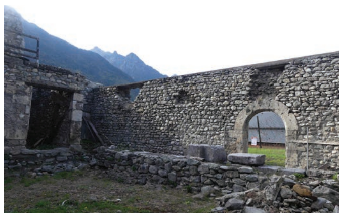
ph6) Mur Nord façade Sud 2019 (D. Perron)
