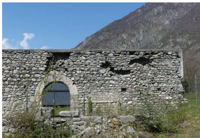
ph9) Mur Nord façade Sud 2022 (D. Perron)
