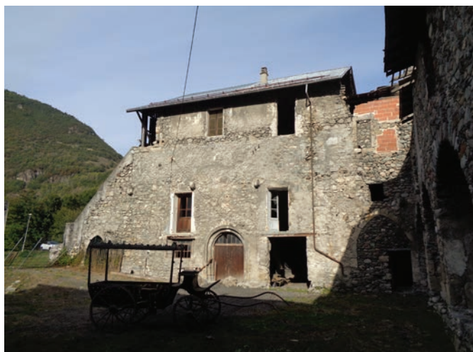
ph38) Mur Nord façade Sud 2010 (D. Perron)
