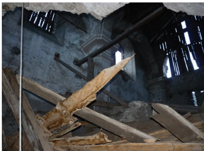
ph91) tribune effondrée 2010 (D. Perron)
