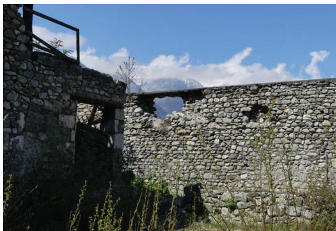
ph8) Mur Nord façade Sud 2022 (D. Perron)
