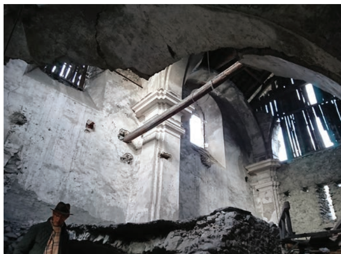
ph92) tribune effondrée 2016 (D. Perron)
